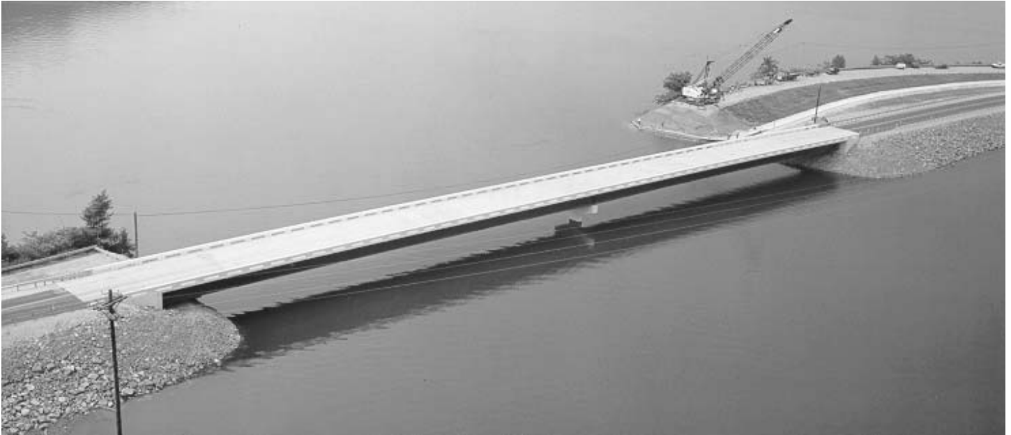
Figure 4. Girders for highway bridges such as this one require multi-pass CJP groove welds.
